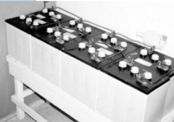
Figure 2.6. A bank of deep-cycle, lead-acid batteries provide energy to operate a vaccine refrigerator 24 hours per day. Photovoltaic panels or a wind generator can recharge the batteries.
