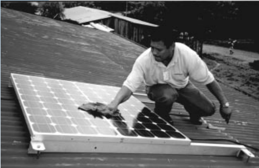
Figure 2.2. A photovoltaic technician cleans two 80-watt panels which power a Sunfrost vaccine refrigerator in the community of Mulukuku, Nicaragua.
